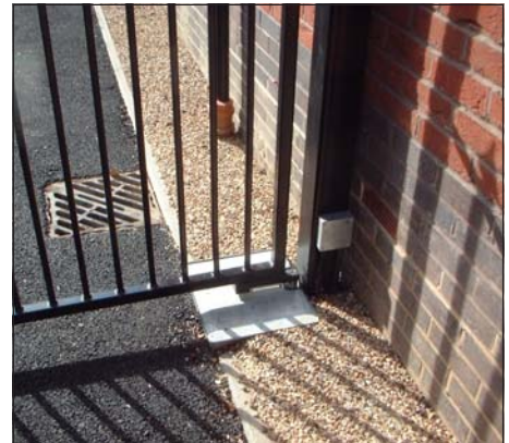
This 'closing gap' between gate and wall is a potential trapping point.
